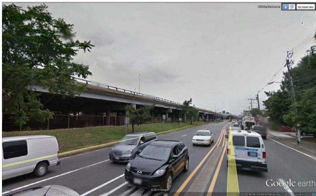
FIGURE 16 Viaduct Approaching Interchange 28/Sullivan Square Exit View Looking South from Mystic Avenue
