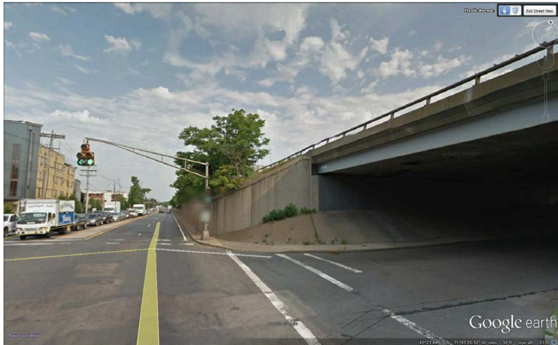
FIGURE 15 Embankment Approaching Interchange 28/Sullivan Square Exit View Looking North from Mystic Avenue
