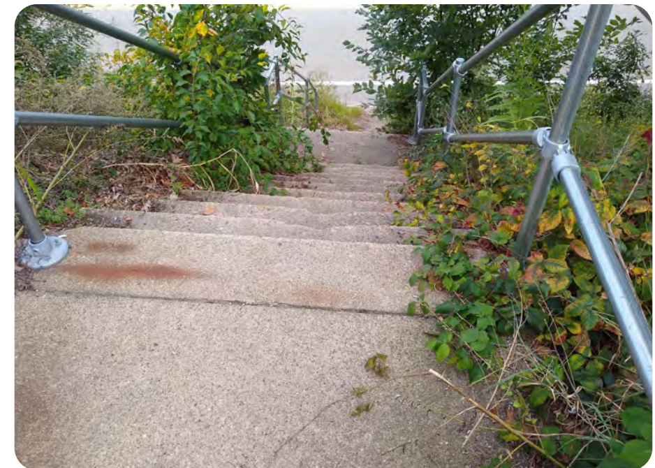
Deteriorating staircase on Concord Street at Route 9
