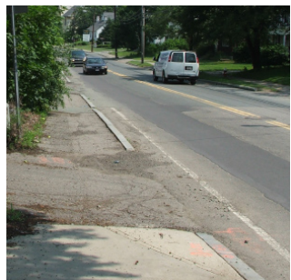
Some of the sidewalks near the study boundary are in need of repair.
