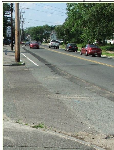
Recent utility work has made the roadway surface along North Franklin and South Franklin streets very uneven.
