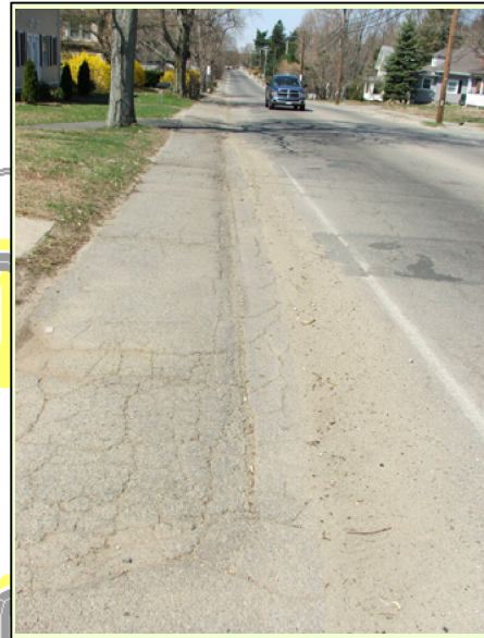
Beyond the immediate town center area, the shoulders contain debris that could be hazardous to bicyclists.
