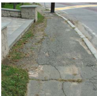
Most sidewalks have bumps and cracks, making them uneven.
