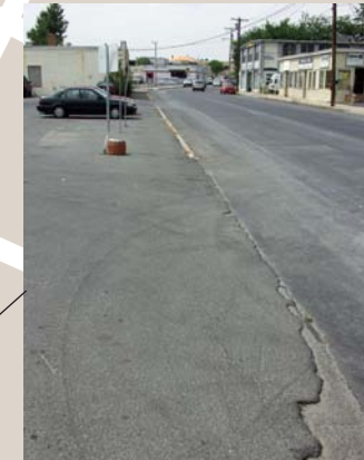
Lack of sidewalk separation
