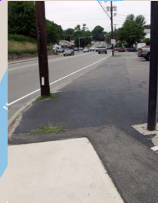
New curb ramps but no sidewalk separation
