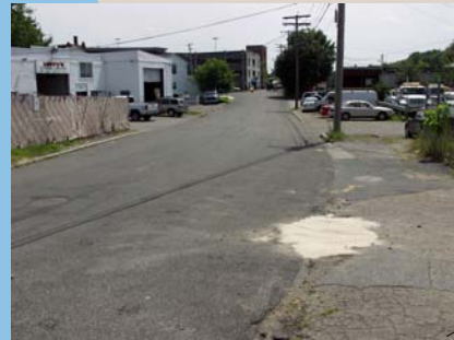
Lack of sidewalks
