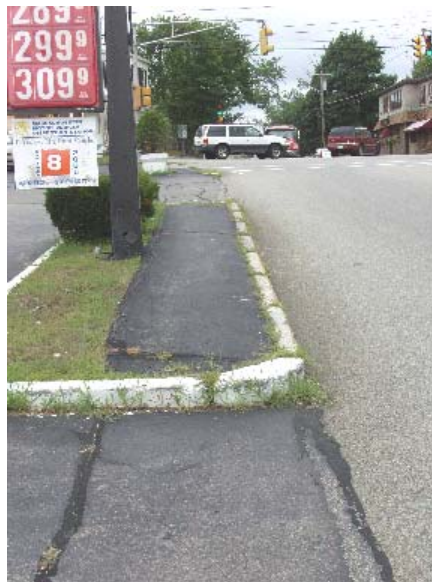
Lack of curb ramps along Broad Street; the Middle Street intersection is in the background
