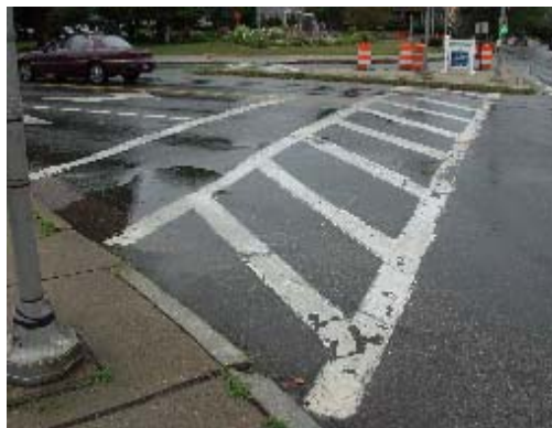
Intersection of Main and Pleasant Streets: no curb ramp, pole obstructing crosswalk.
