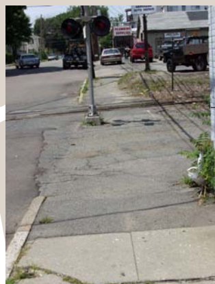
Disrepair near railroad tracks
