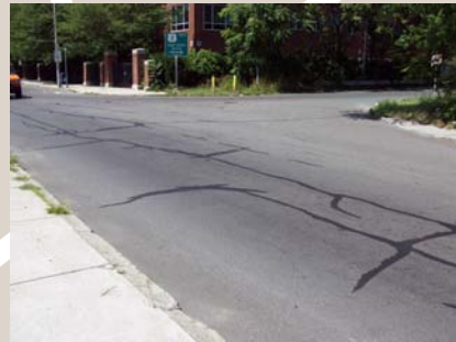
Lack of crosswalks
