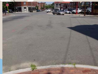
No markings to guide motorists through intersection
