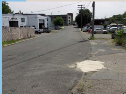
Lack of sidewalks
