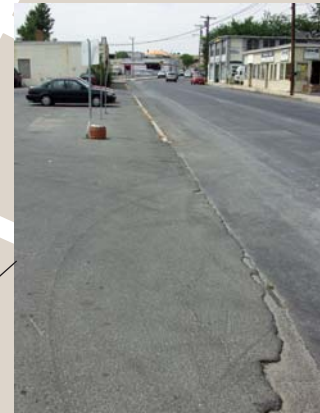
Lack of sidewalk separation
