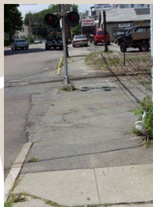
Disrepair near railroad tracks
