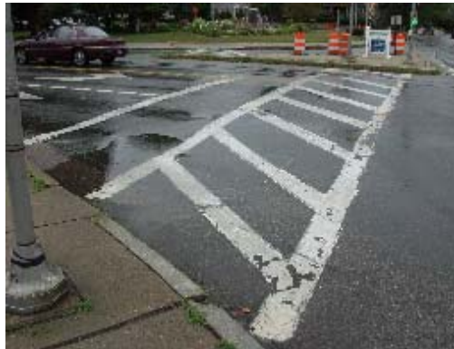
Intersection of Main and Pleasant Streets: no curb ramp, pole obstructing crosswalk.
