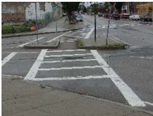
Misaligned crosswalk across Summer Street
