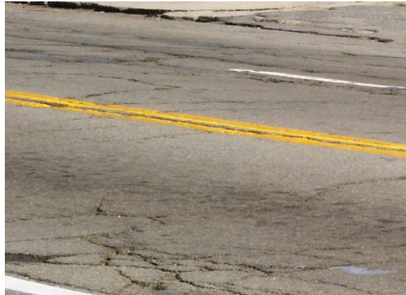
Morton Street, west of Blue Hill Avenue: pavement is broken.
