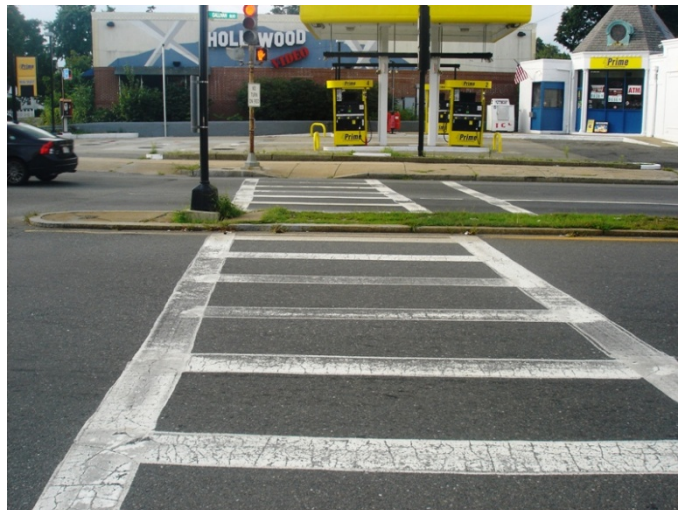
Gallivan Boulevard at Granite Avenue/Adams Street: No opening in the median to connect the crosswalks
