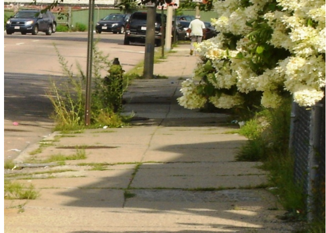
Morton Street, west of Norfolk Street: Sidewalk broken and vegetation has reduced the effective width of the sidewalk
